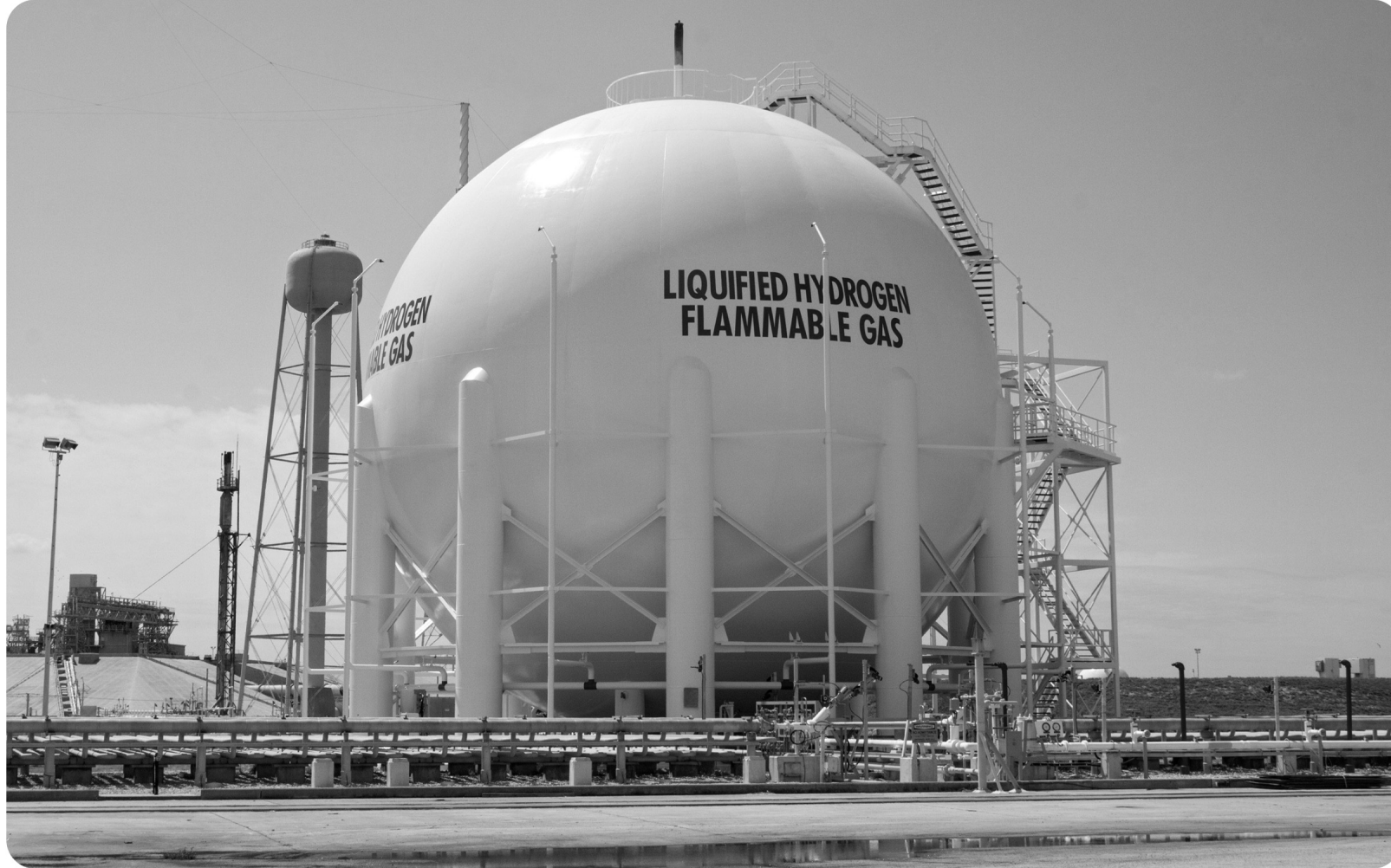
Liquid hydrogen storage. FSEC®. (2018, July 6). [Image] Retrieved from https://energyresearch.ucf.edu/research/hydrogen/liquid-hydrogen-storage/
