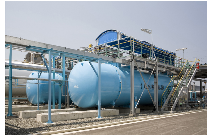
Cryogenic Tank for Hydrogen Liquefaction [10]
