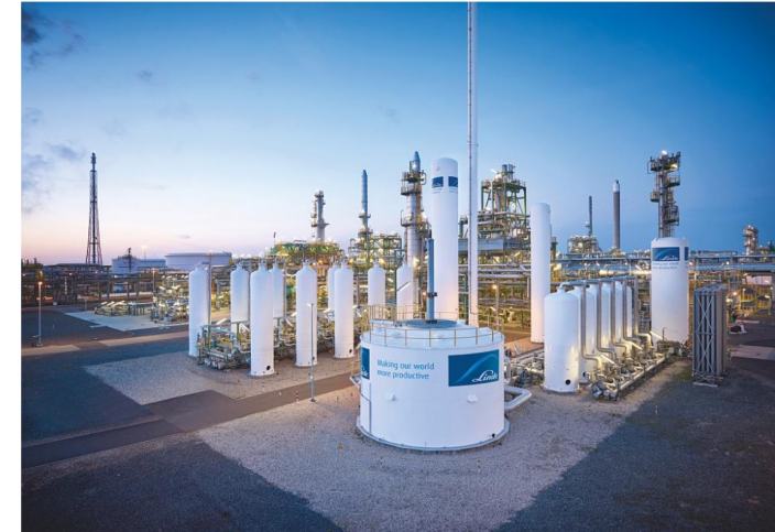
Leuna Hydrogen Liquefaction Plant in Germany [9]
